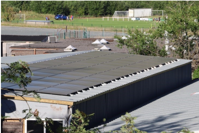
Our bank of solar panels
