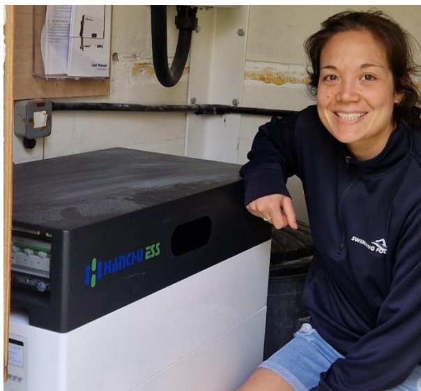
Pool manager Tash Ward with the new batteries
